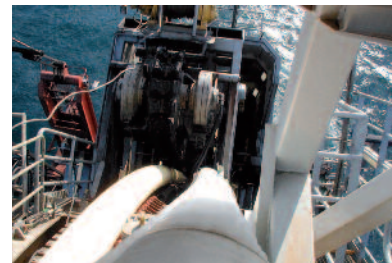
Pipe & DEH CPS Firing Line
